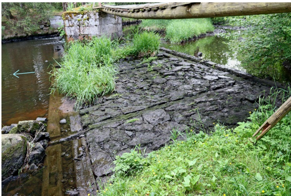
Fig. 8. Blansko near Kaplice, the Ponzholz barrier, the reinforced riverbed below the barrier, downstream direction, indicated flow direction, photo: Marie Hansová, 2024
